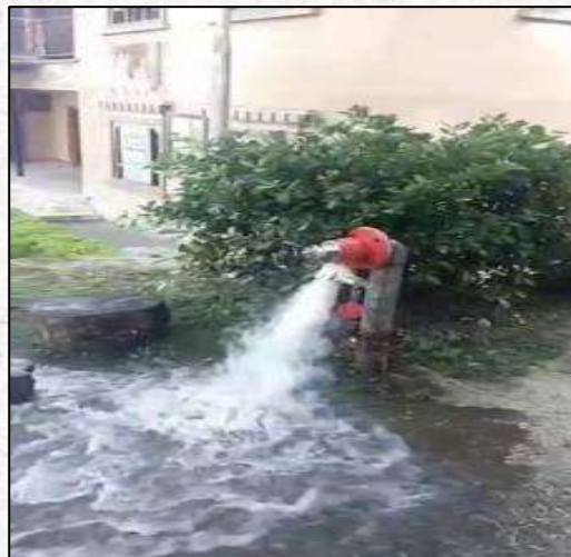
Fire Hydrant at Mongar School
